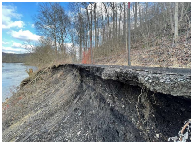
Blackhand Gorge State Nature Preserve Trail Slip Before Repair
