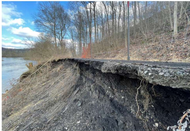
Blackhand Gorge State Nature Preserve Trail Slip Before Repair
